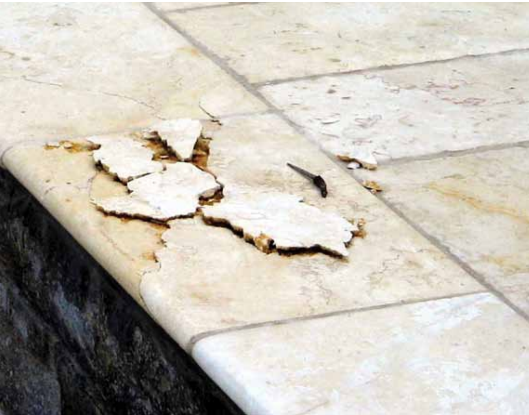
Degradation due to saturated freeze/thaw cycling of a limestone cap
